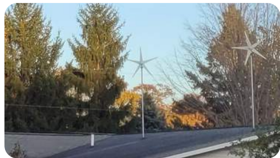
Rooftop-mounted wind generators on a home in Breitung Township
